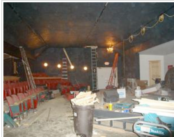
The Northport Music Theater, very much a work in progress in January ...
